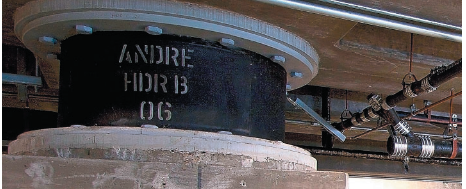
Mounted on massive “base isolator” shock absorbers, our data centers can survive earthquakes many times the magnitude of the 1906 San Francisco quake.
