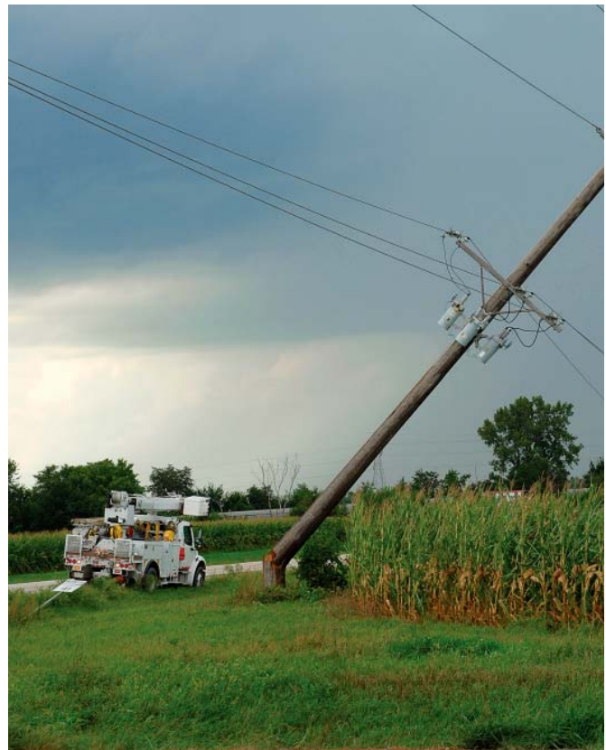
CoreLogic Natural Hazard Risk Layers help telecoms analyze and manage risks and emergencies.
